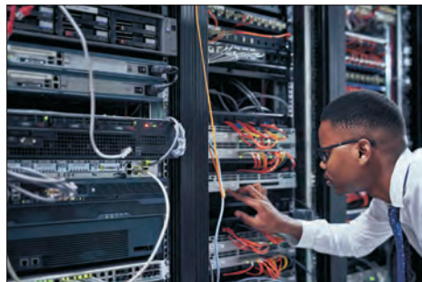
A technician working and checking if all servers are up and running. Photo via iStock.com/PeopleImages. [Used under license.]
